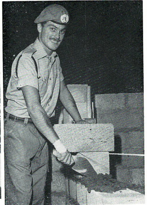
Building a wall of a new accommodation block at one of the OPs.
